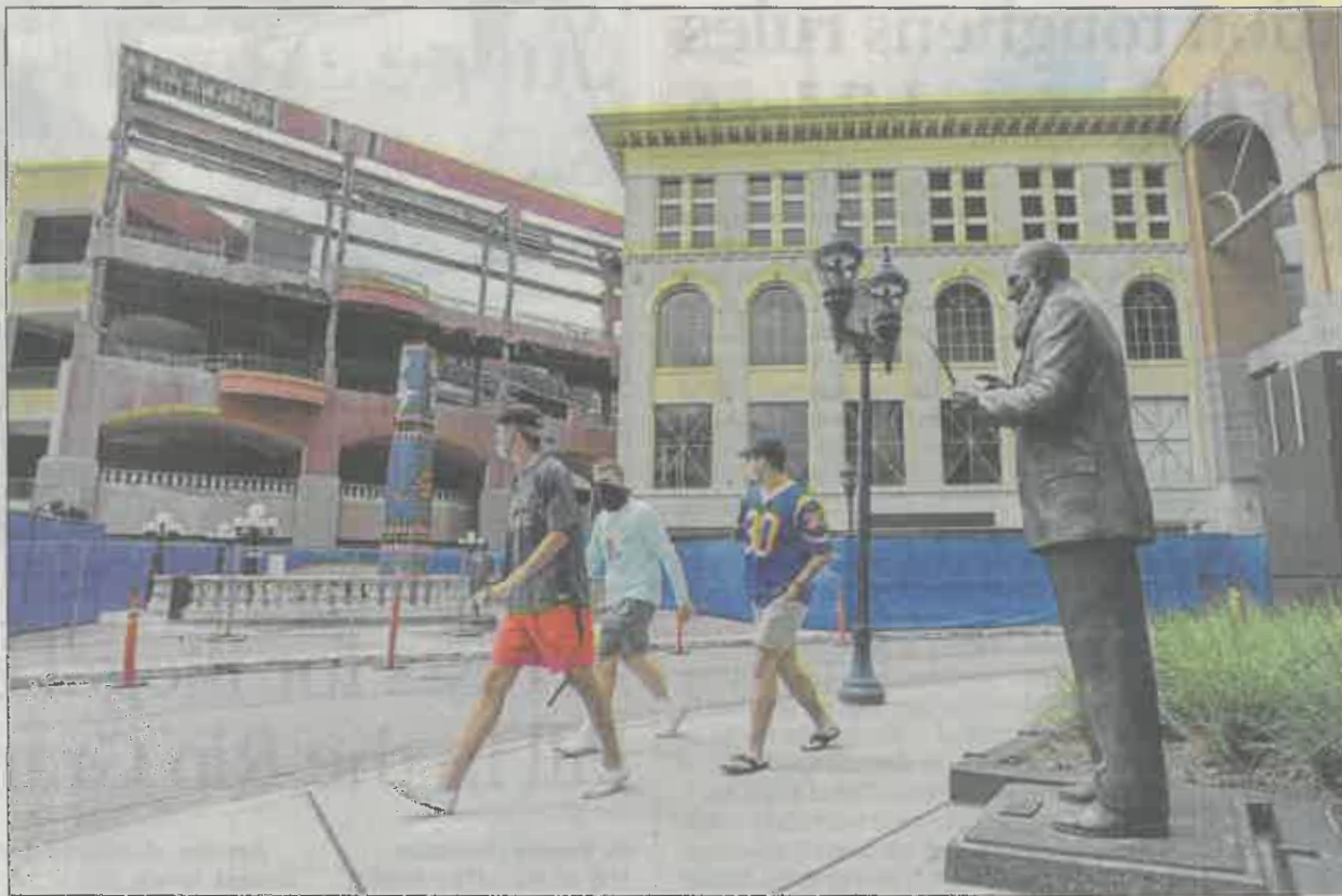
Crews work to demolish Horton Plaza, at left, in June 2020. The lender behind developer Stockdale Capital Partners' Campus at Horton has started the foreclosure process to recoup $351.2 million in debt. EDUARDO CONTRERAS / U-T FILE
